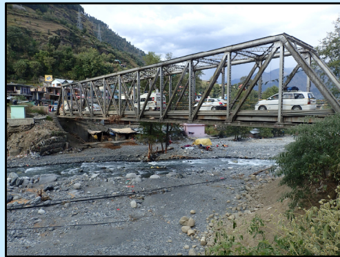
Fig. 2: Sept. 2018 flood impacts in Phojoal Nalla (near Katrain) bringing significant channel change and destruction of forestry, horticulture, electricity transmission networks, roads, bridges & buildings
